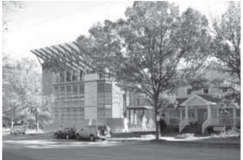
Southface Eco Office is a 10,000-square-foot commercial demonstration center that will help architects, builders, and developers learn easy ways to save energy, conserve water, and preserve the environment. Currently it's under construction, and tracking for LEED-Platinum certification. Architect: Lord, Aeck & Sargent.
